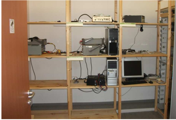
Part of the Server Room
